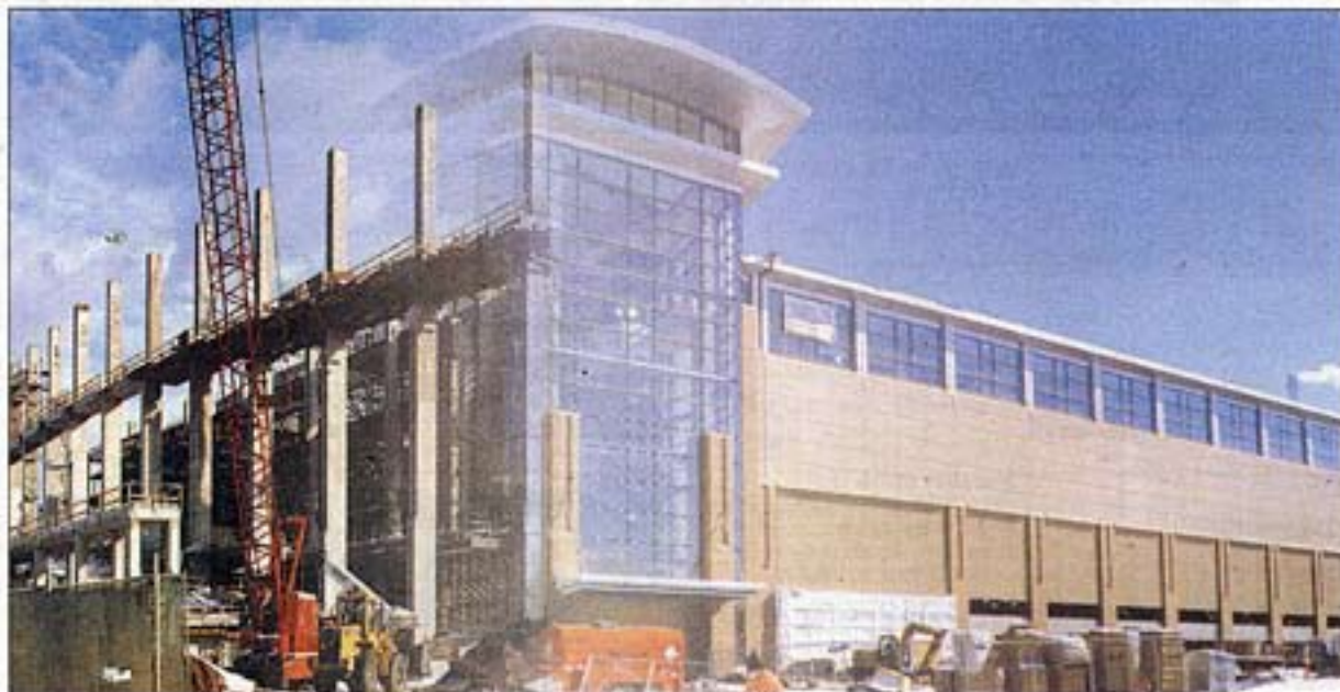
Many of Manafort Brothers buildings dot the Connecticut skyline, such as the Connecticut Convention Center in Hartford.
