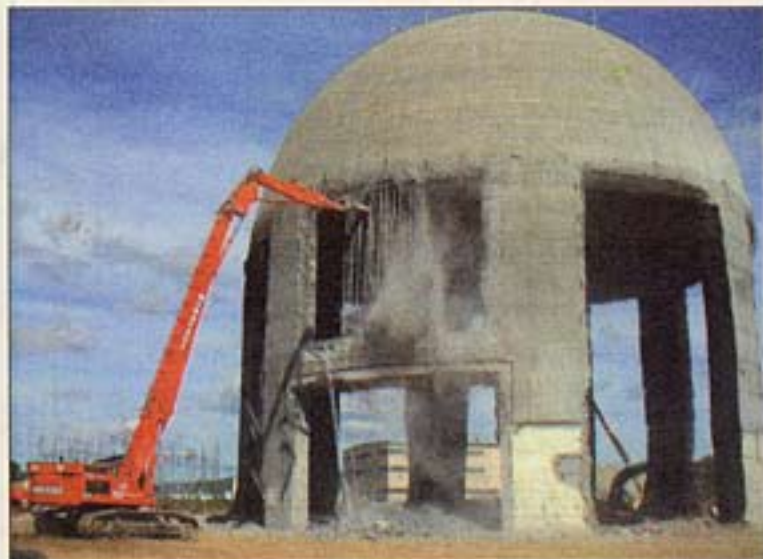
The Manafort Brothers are experts in very tricky work, such as the construction of the Maine Yankee Nuclear Power Plant in Wiscasset, Maine.
